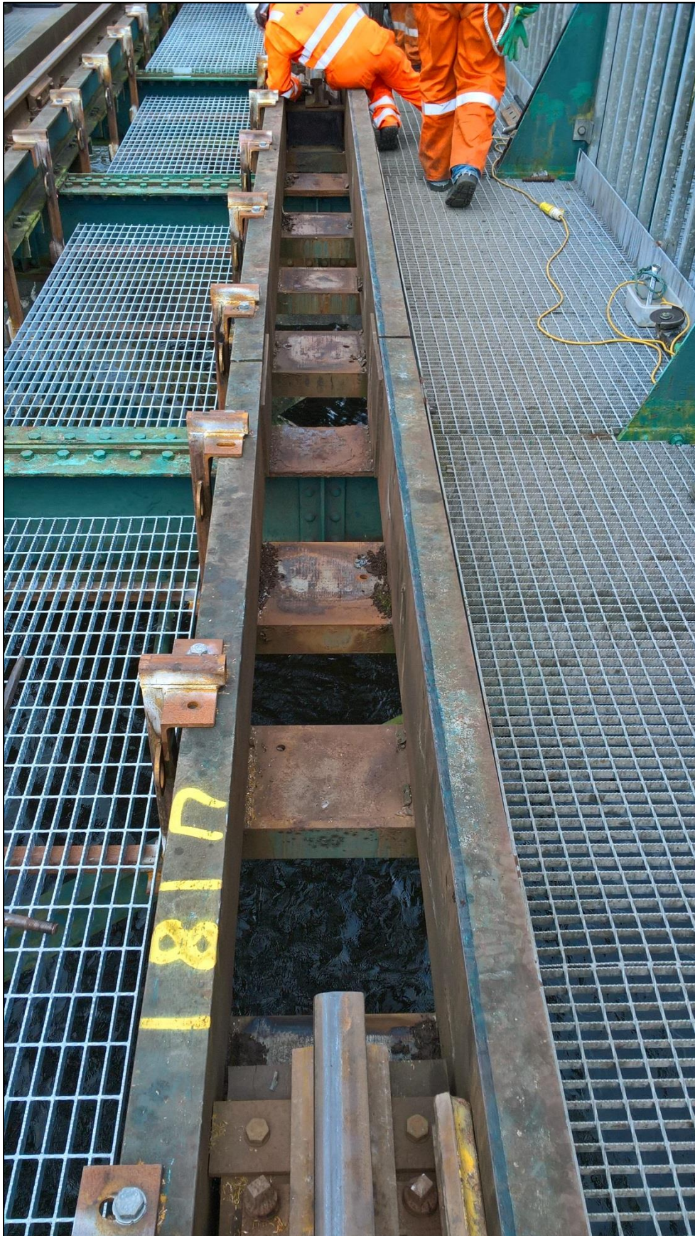
Photo 3. Shows waybeam removed at UBE16 illustrating how the waybeam is supported at intervals.
