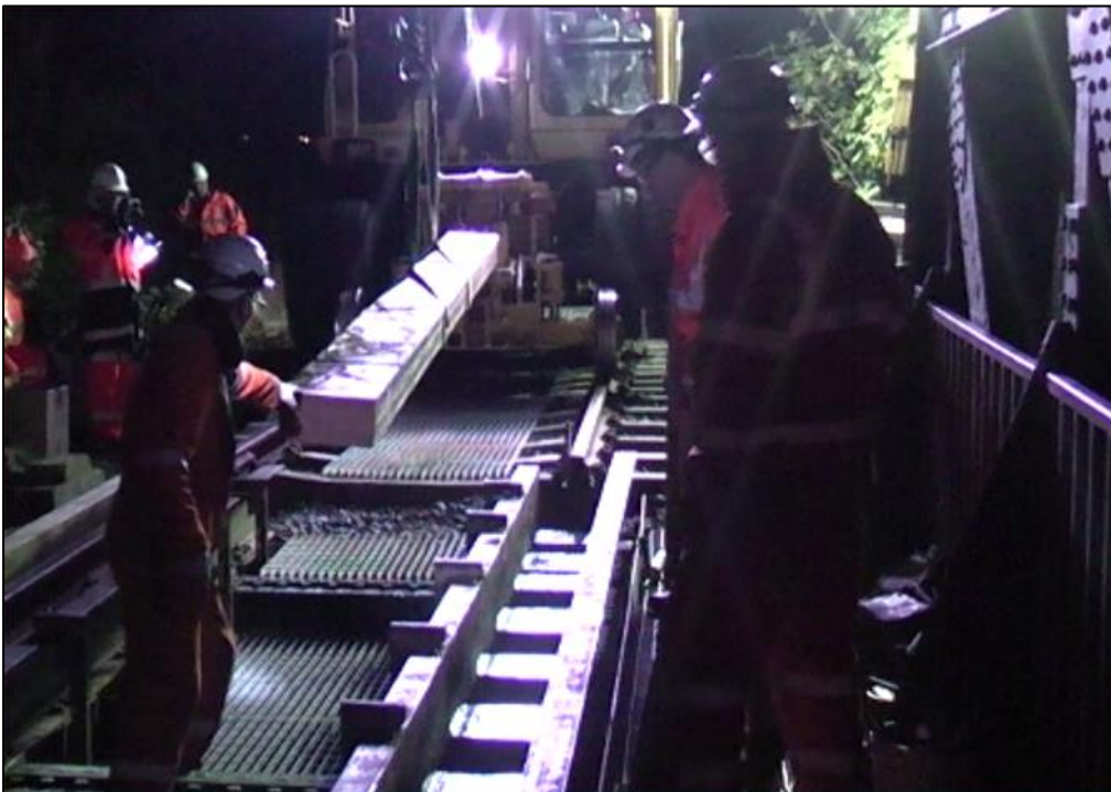
Photo 5. Renewal of the waybeams with FFU commenced during night working in September.
