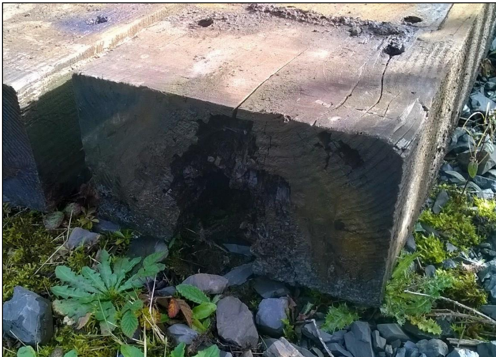
Photo 2. View showing rot in timber waybeam removed from UBE16. Note how there is no visual indication on the top surface of this deterioration.
